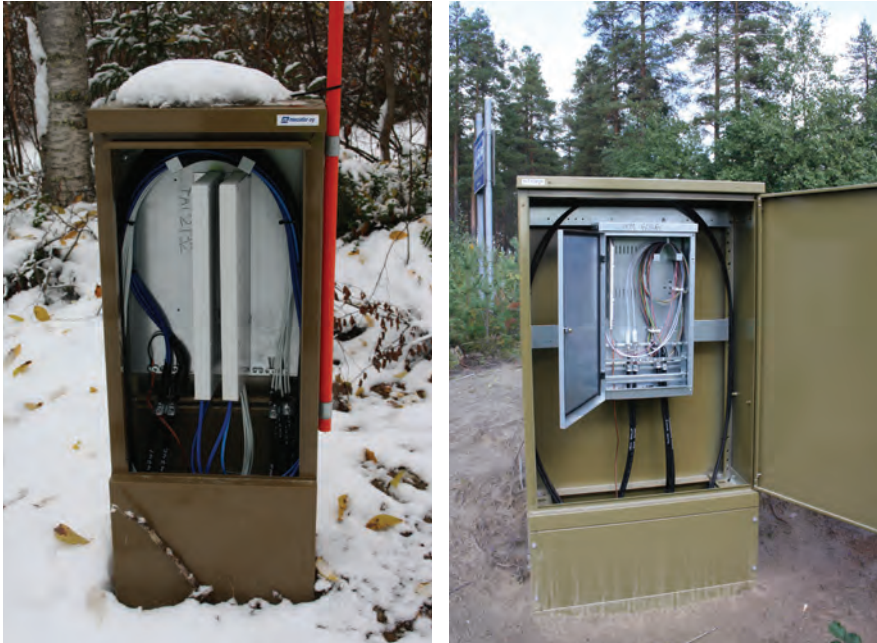
Figure 4.23. Splice cabinets in their installation environment.
