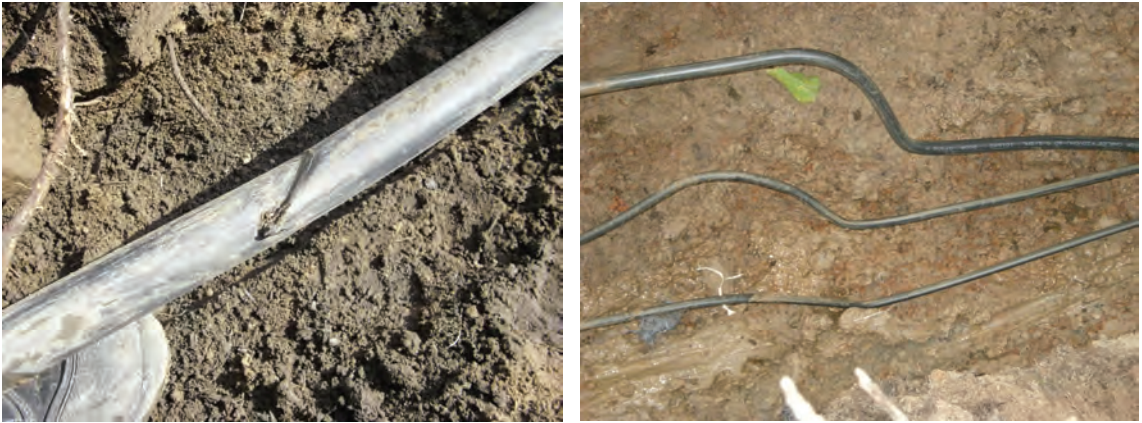
Figure 10.2. Examples of cable faults.
