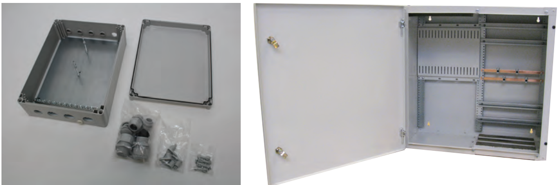
Figure 4.24. Example of an indoor joint closure and splice cabinets.
