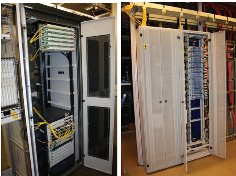
Figure 4.20. Examples of optical fibre distribution racks used in an optical access network.
